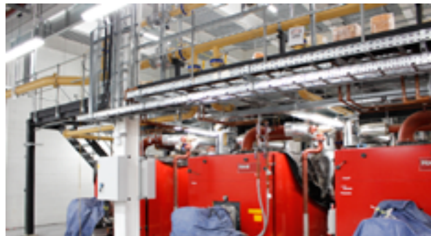
Electrical equipment located within the Energy Centre
