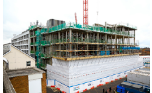
External shot of the Acute Services Block progress at five storeys high
