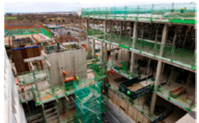
Work on the New Ward Block underway with concrete and scaffolding in place
