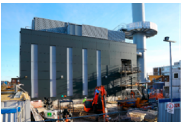
External shot of the Energy Centre
